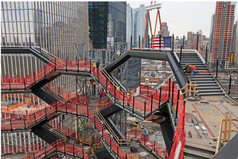
The topping out of Vessel . Courtesy of Related Companies and Oxford Properties.
